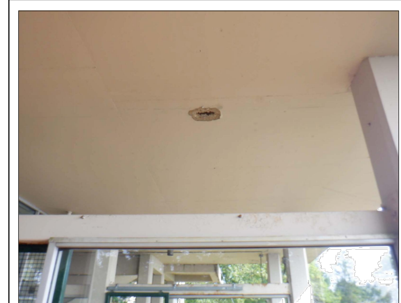
STANDING ON LOADING PLATFORM NO. 2 AND LOOKING UP AT HOLE ON THE UNDERSIDE OF THE OBSERVATION DECK ABOVE CARS
