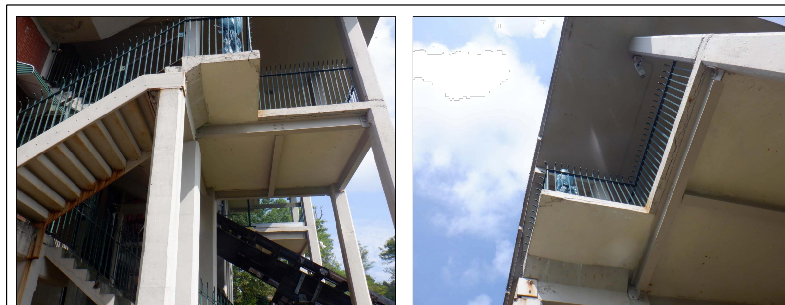
STANDING ON THE GROUND AND LOOKING UP AT LOADING PLATFORM NO. 2 SHOWING SLAB CRACKING
