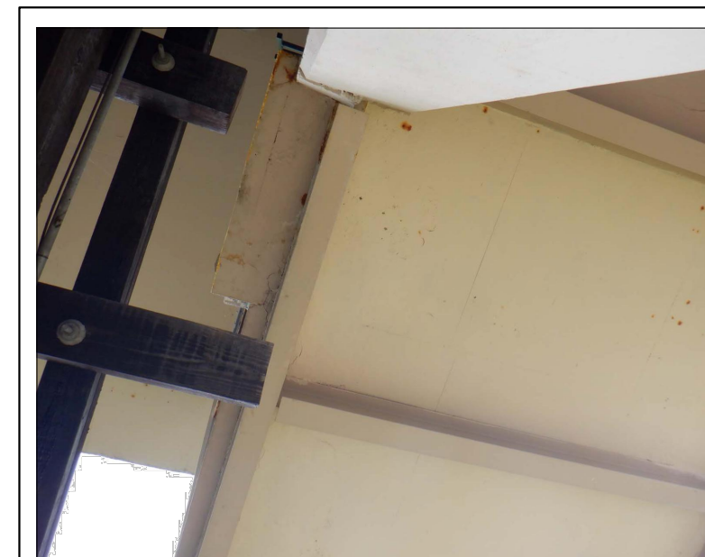
STANDING ON THE GROUND AND LOOKING UP AT UNDERSIDE OF LOADING PLATFORM NO. 2 DOORWAY
