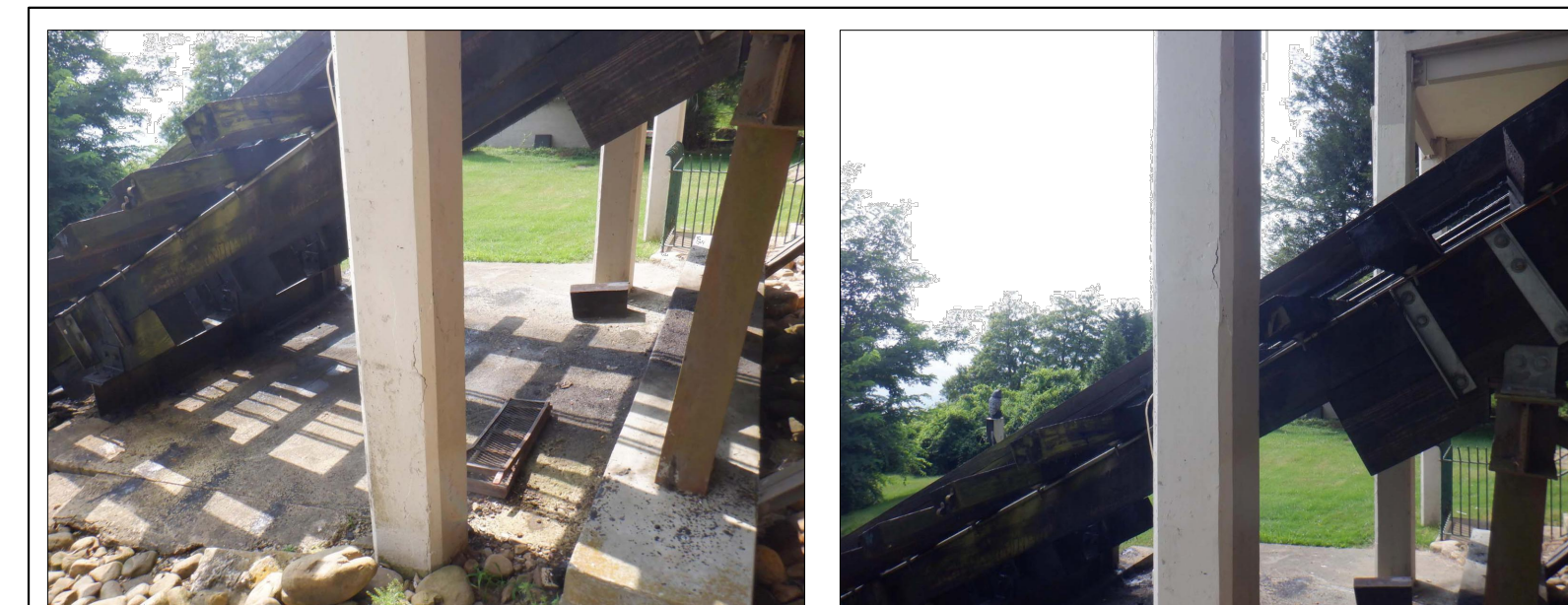
STANDING ON LOADING PLATFORM NO. 2 STEPS AND LOOKING AT UNDERSIDE OF STEPS LEADING TO OBSERVATION DECK SHOWING CONCRETE SPALLING
