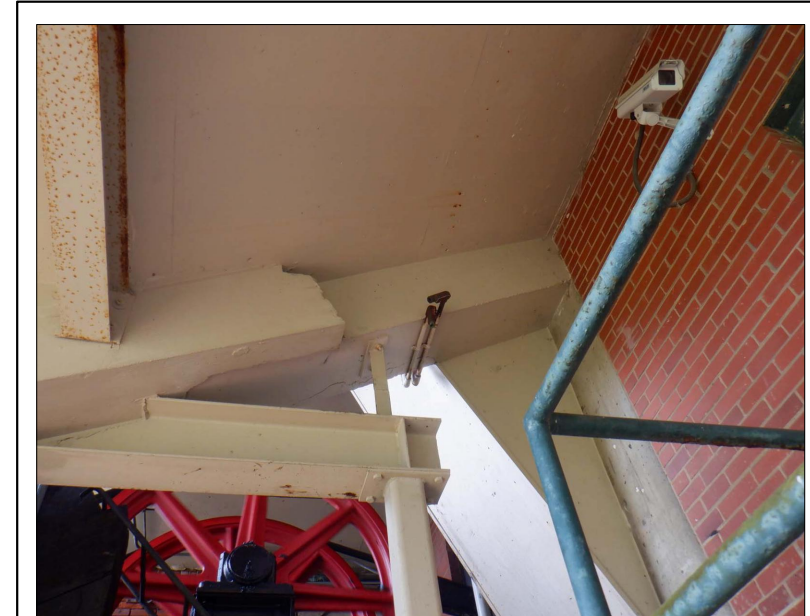
STANDING ON THE GROUND AND LOOKING UP AT UNDERSIDE OF LOADING PLATFORM NO. 2 DOORWAY
