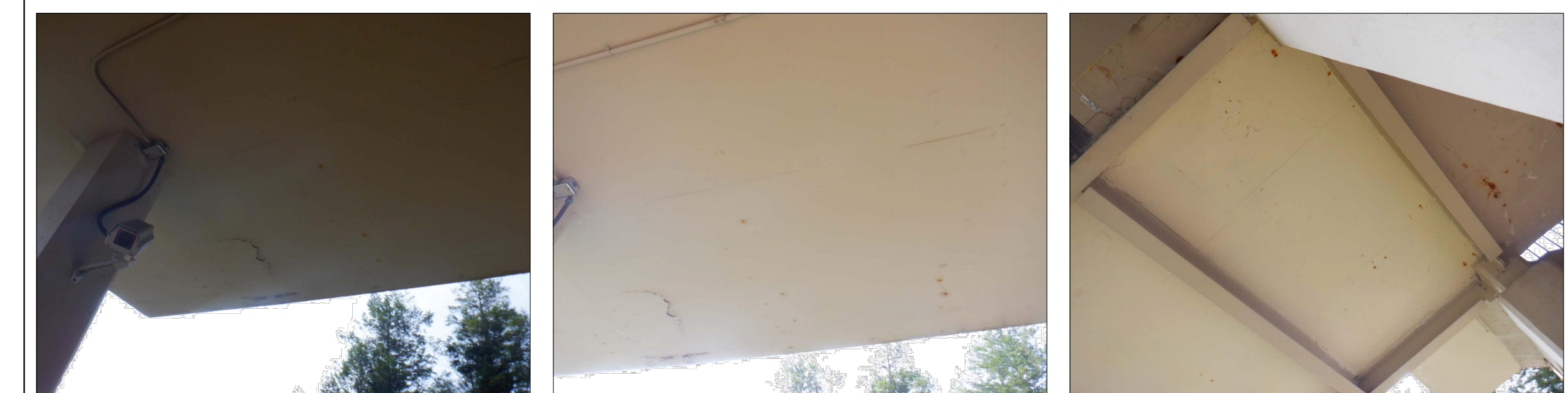
STANDING ON LOADING PLATFORM NO. 2 STEPS AND LOOKING SIDE OF LANDING SHOWING CONCRETE CRACKING
