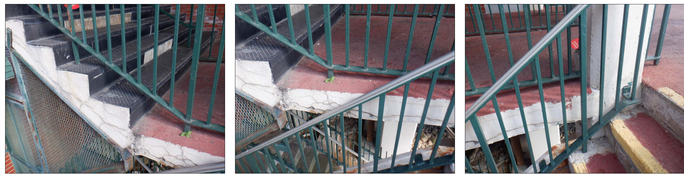
STANDING ON LOADING PLATFORM NO. 2 STEPS AND LOOKING SIDE OF LANDING SHOWING CONCRETE CRACKING
