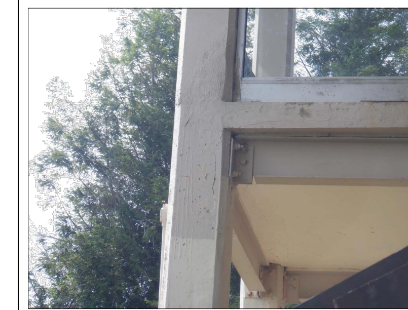
STANDING ON LOADING PLATFORM NO. 1 AND LOOKING AT SIDE OF SLAB OF LOADING PLATFORM NO. 2 CRACKING AND VERTICAL CRACK IN COLUMN
