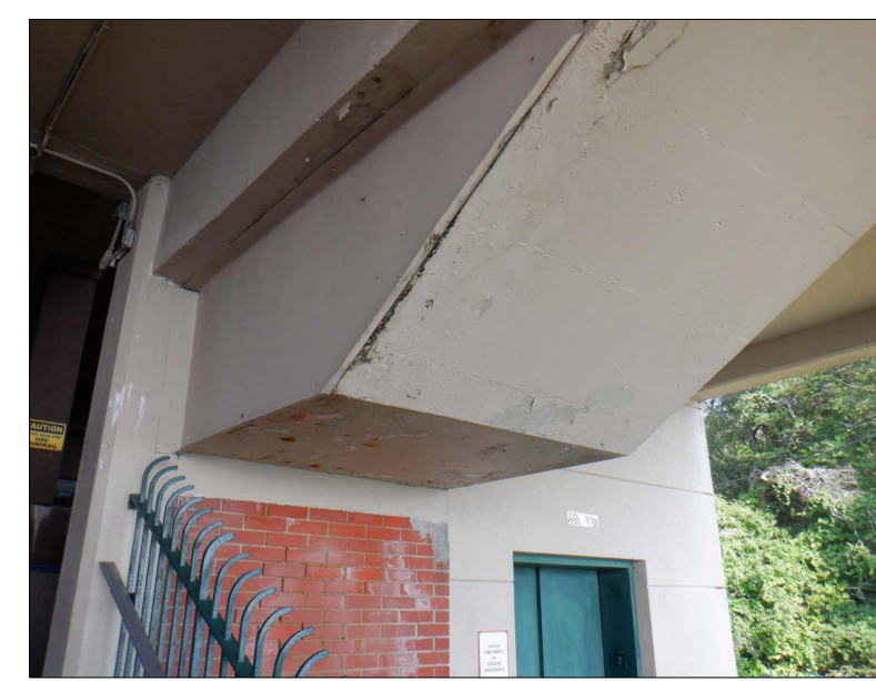
STANDING ON STAIRS LEADING TO LOADING PLATFORM NO. 1 LOOKING UP AT DELAMINATION ON UNDERSIDE OF STAIRS LEADING UP TO THE OBSERVATION DECK
