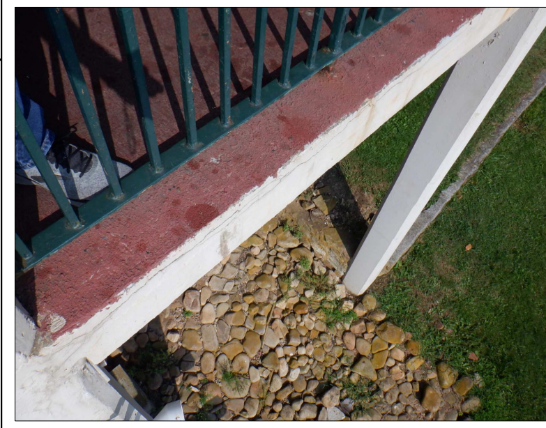
STANDING ON LOADING PLATFORM NO. 1 AND LOOKING AT SIDE OF SLAB OF LOADING PLATFORM NO. 1 CRACKING AND DELAMINATION
