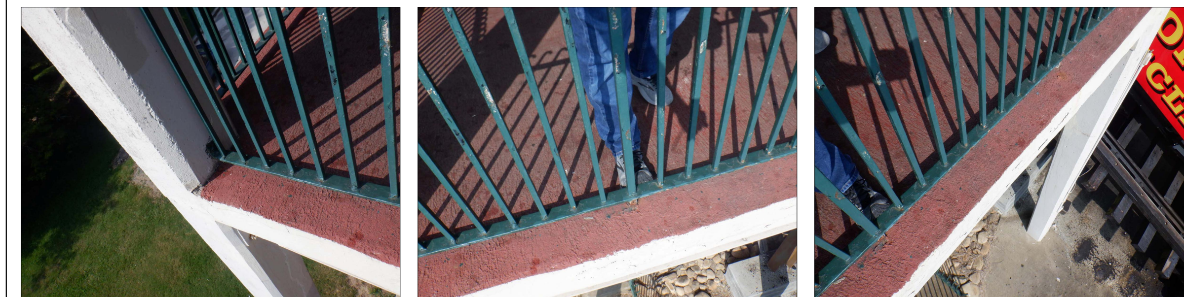
STANDING ON LOADING PLATFORM NO. 2 AND LOOKING AT SIDE OF SLAB OF LOADING PLATFORM NO. 2 CRACKING AND DELAMINATION
