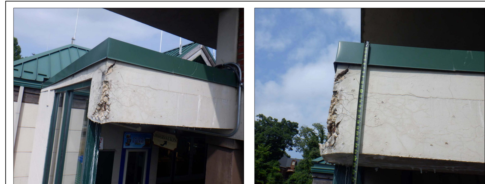
STANDING ON STEPS LOOK BACK AT DAMAGED BEAM
