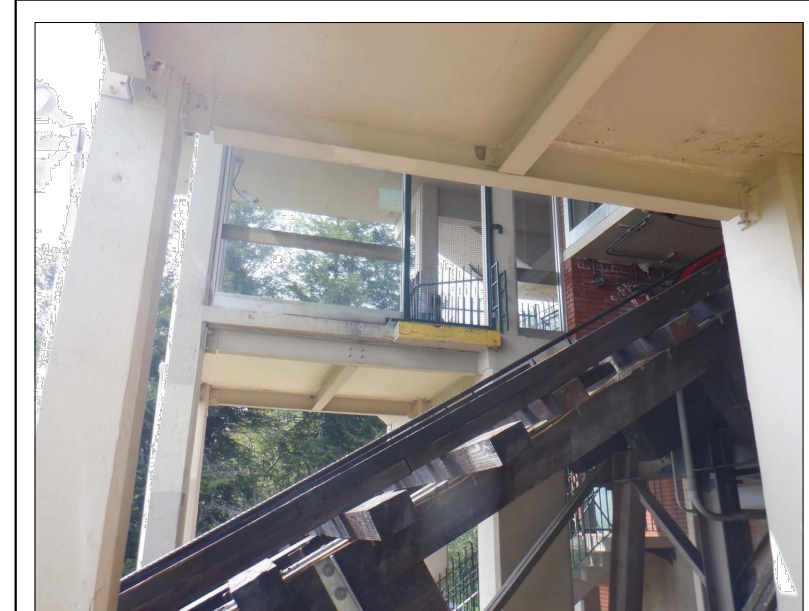
STANDING ON THE GROUND AND LOOKING UP AT CRACKING ALONG THE EDGE LOADING PLATFORM NO. 2
