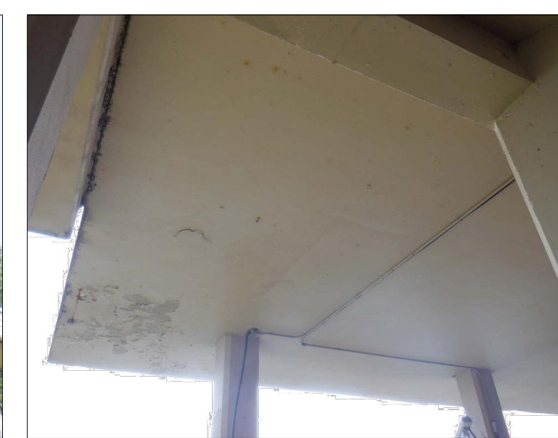
STANDING ON ELEVATOR PLATFORM LOOKING UP AT SPALLING AREA ON UNDERSIDE OF THE OBSERVATION DECK
