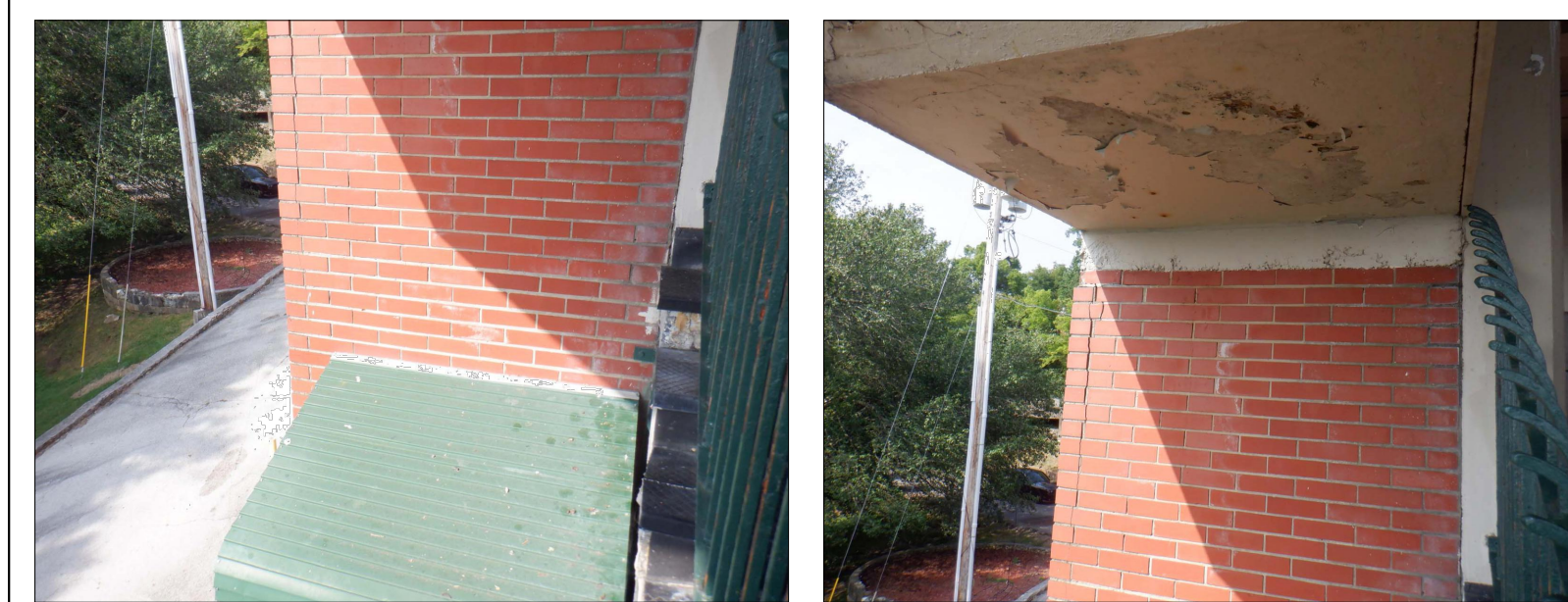
STANDING ON STEPS AND LOOKING AT THE CORNER OF THE BUILDING SHOWING VERTICAL CRACKING IN THE BRICKS
