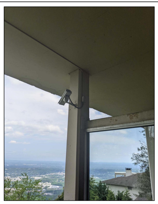
LOOKING AT A CAMERA IN STORE FRONT 1 LOCATION THAT MAY NEED TO BE RELOCATED
